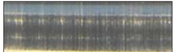
Condition at depth of around 100mm
